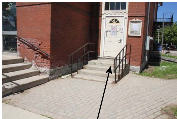
Non-compliant exterior stairs.
