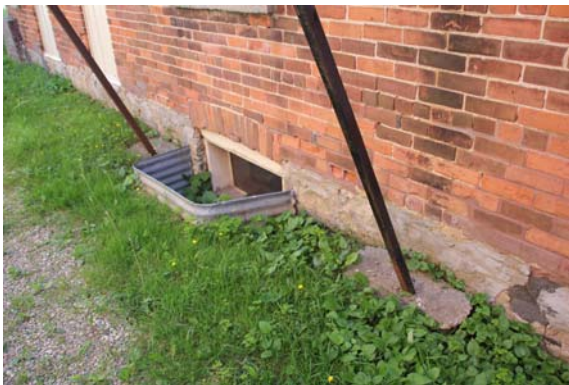
Stone foundation wall requires mortar pointing. Diagonal steel members, supporting fire escapes, are under structured.
