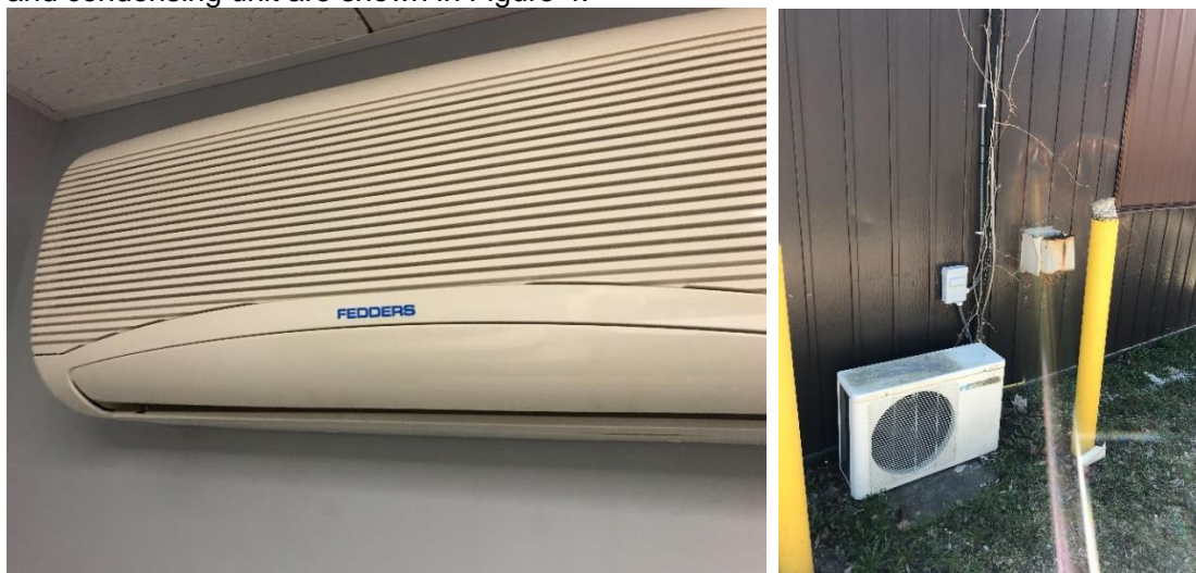
Figure 4: Addition Air Conditioning Unit
