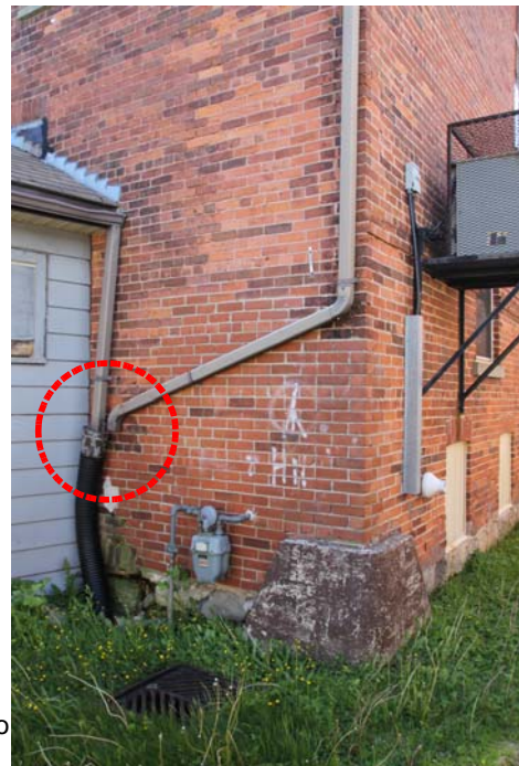
Rainwater leaders are not connected to drain pipe resulting in saturation of wall masonry and deterioration of foundation wall. This area of wall has been subject to previous repairs.
