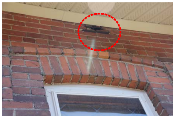
Ends of steel trusses are visible at building exterior. Note that this truss bears directly over wall opening for window.
