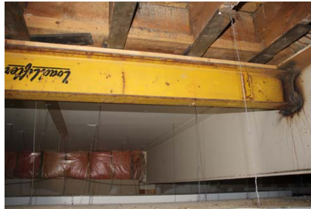
24" deep (white coloured) steel beam spans width of building, supporting 2 nd floor structure. Yellow beam was added to support failed wood beam directly above.
