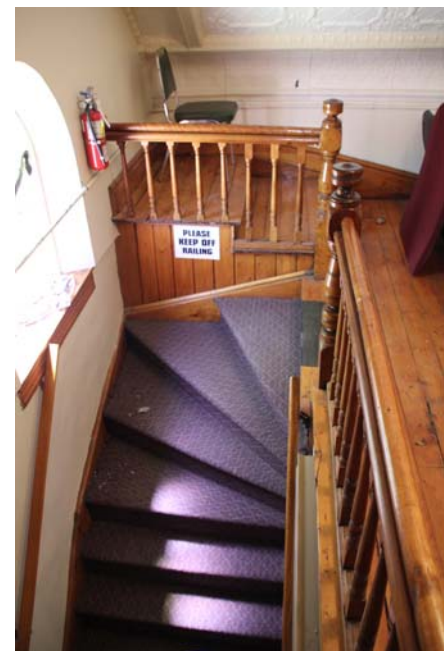
Balcony stair with curved winders and non-complaint guard around balcony opening.
