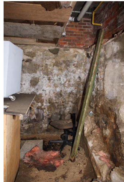
Northwest basement corner is very damp due to disconnected exterior rainwater leader draining eave gutter. Note the accumulation of mortar fines primarily at toe of foundation wall.
