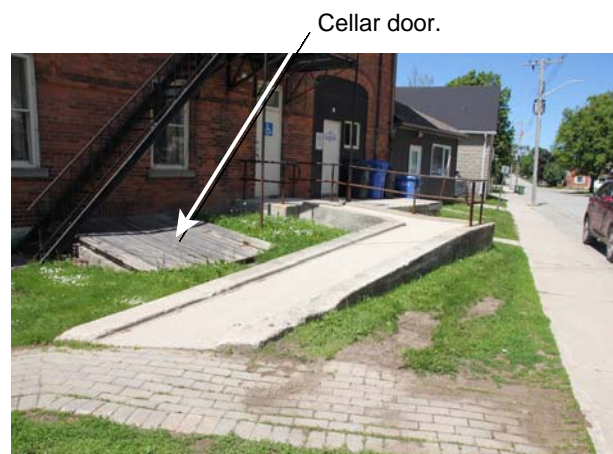
Non-compliant exterior concrete ramp.
