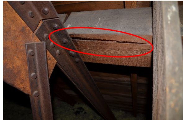
Purlin Connection @ Truss Purlin split at bolted connection
