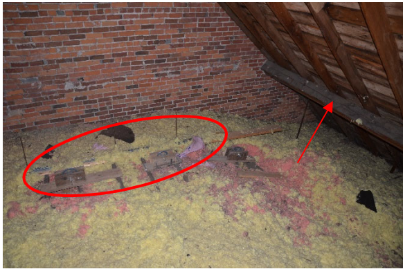
Framing over Elevated Performance Platform No additional support at rigging locations Purlins sagging
