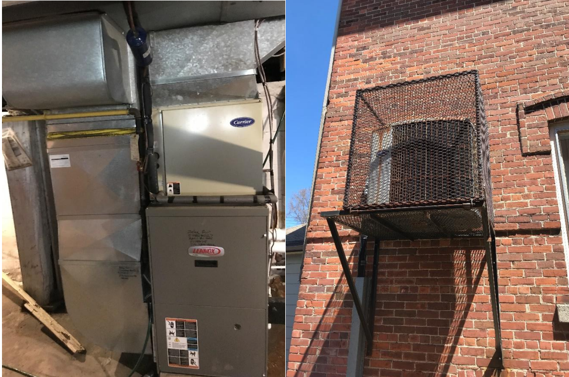
Figure 2: Furnace and Condensing Unit
