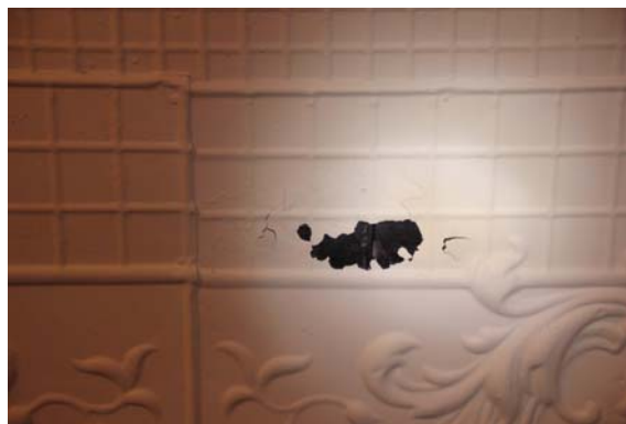
Peeling paint, from underside of performance hall pressed metal ceiling, must be tested to determine if paint contains lead. Paint debris should be assumed to be lead containing until testing proves otherwise.
