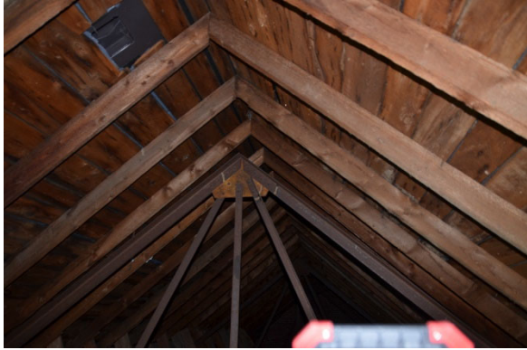
Roof Framing – no collar ties
