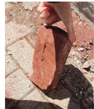
Brick units were heavy with moisture but in reasonable condition.
