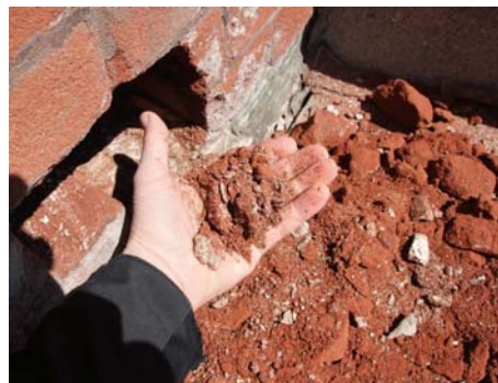
Mortar removed from joint is moist enough to clump and hold under hand pressure.
