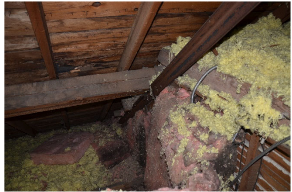
Transition from Attic floor to Elevated Performance Platform Area Ceiling/floor joists bear on purlins
