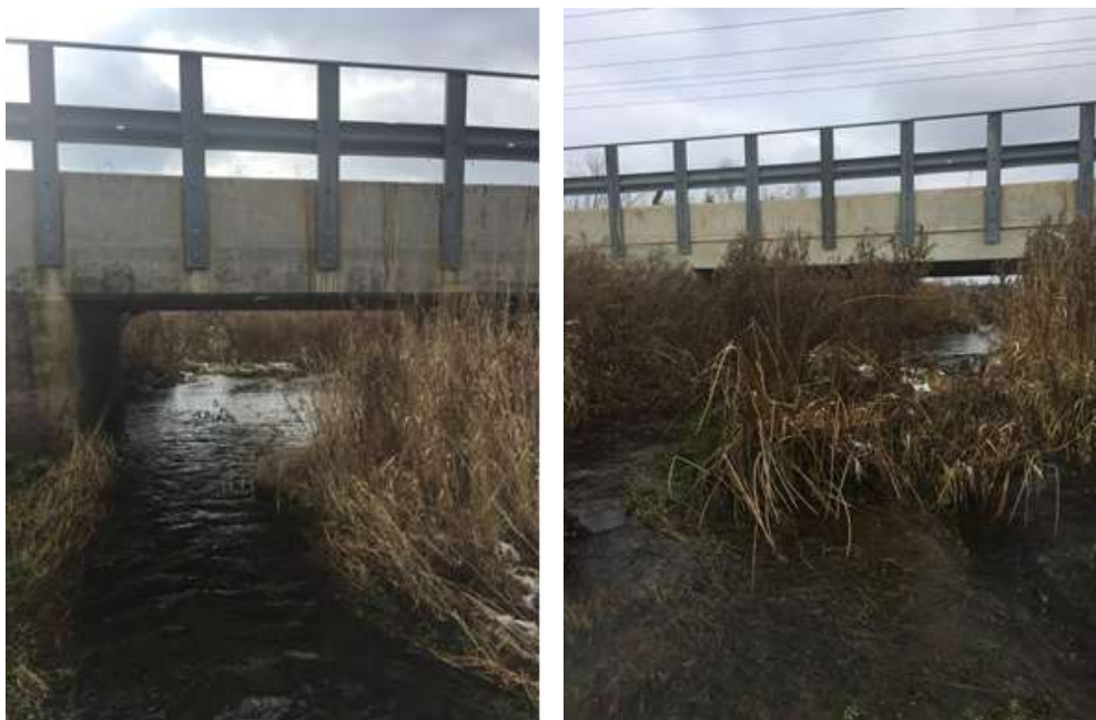
Plate 1: View of channel of James Foley Drain at bridge on Ida Street. View on left shows the channel upstream of the bridge whereas the view on the right shows the channel downstream of the bridge. This bridge was observed to have approximately 20 active Barn Swallow nests.
