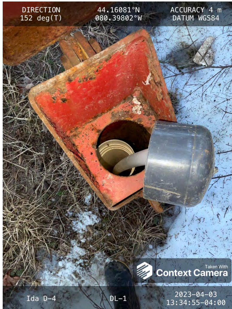
Photo 9: DL-1 with loose cap
